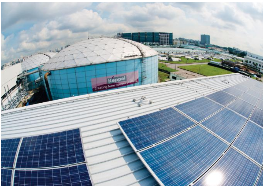
The solar photovoltaic installation at the Keppel Seghers Ulu Pandan NEWater Plant generates up to 1.2 GWh of renewable energy each year.
