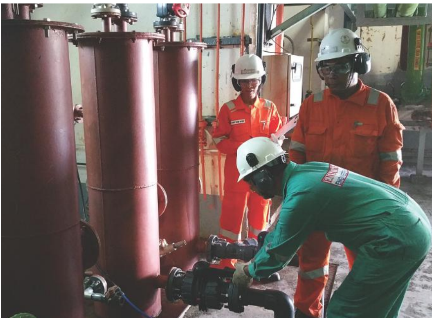
The Senoko WTE Plant O&M team installed an effluent filtration system to reduce the amount of NEWater consumed during dry spells.
