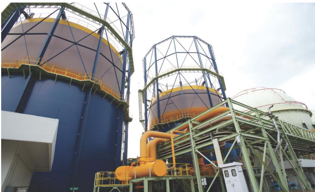
City Gas' production facility, Senoko Gasworks, achieved 100% availability in FY 2016.
