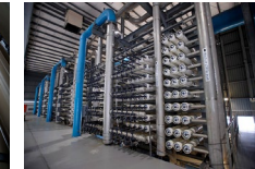
SingSpring Desalination Plant
