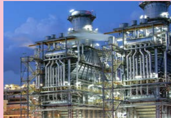
A top-tier gas-fired power plant in Singapore
